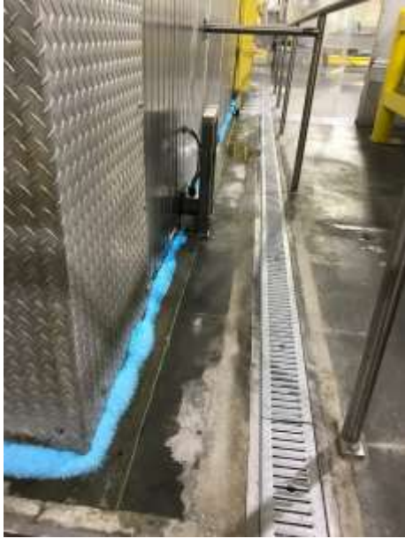
Containment and Monitoring
